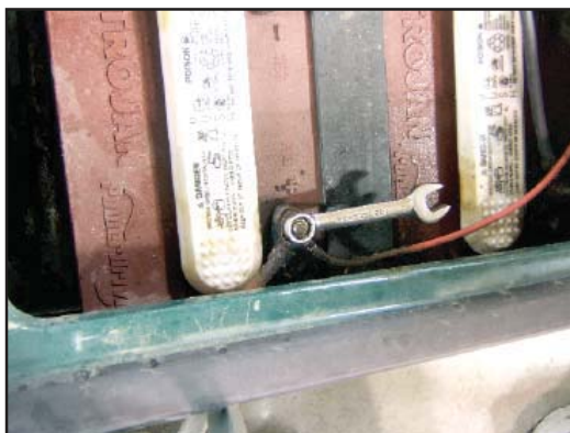
24. Positive Battery Connection
